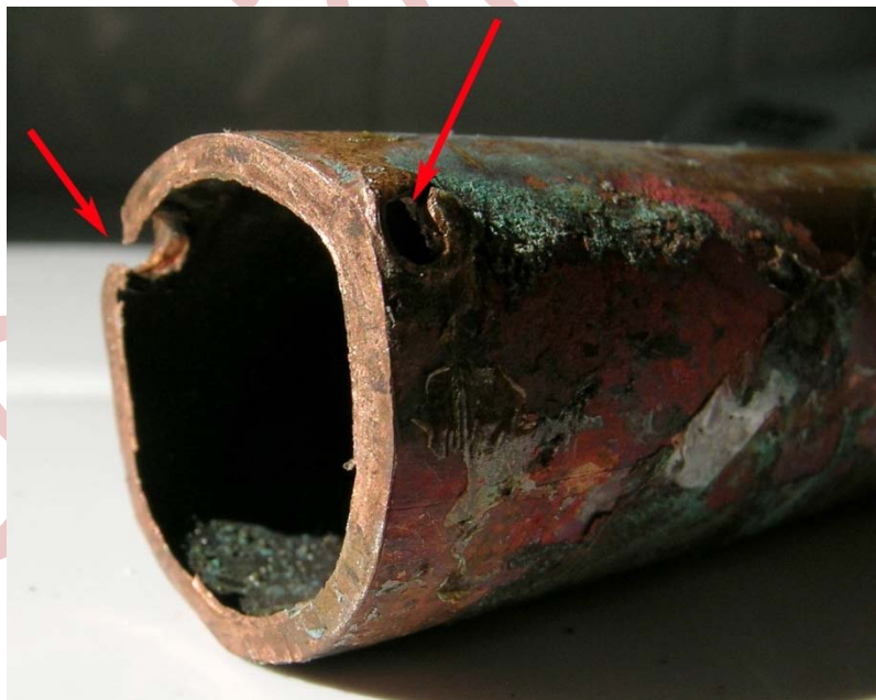
Figure 1. As-received copper pipe. Red arrows represent entry and exit point of wood screw.
