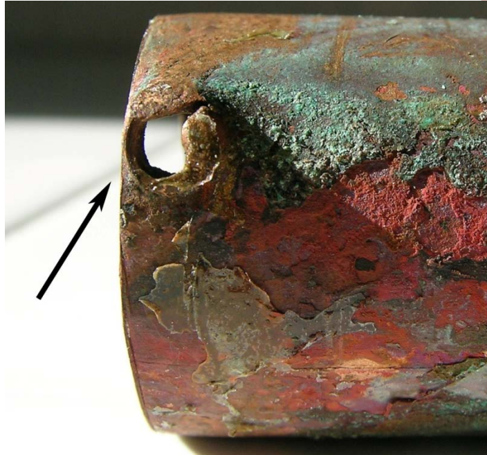
Figure 2. Copper pipe illustrating hole created by wood screw. Note shape of hole reflects deformation created by wood screw penetrating wall of pipe.
